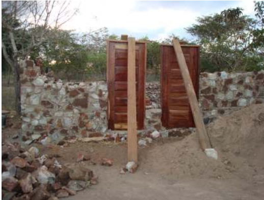
The beginning of our guard's house. So our guards don't have to find shelter in a tent that leaks when it rains.
