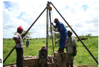
Pulling the old pipping in order for the new pump to be put in place 143 ft deep.
